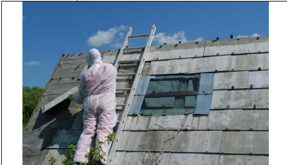
Image 3: Asbestos - Worker on a rooftop
